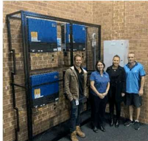
Kiama Leisure Centre - 99.6kW Photovoltaic system.
