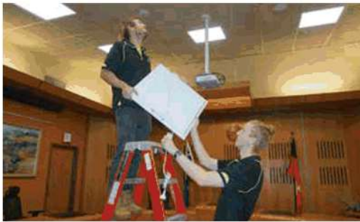
In March 2021, Kiama Council completed an LED lighting upgrade of its administration building.
