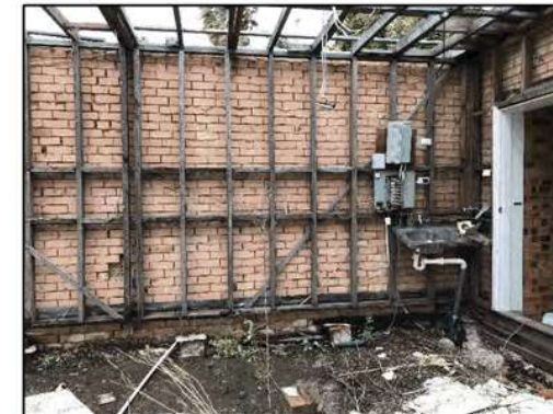
Figure 29. View to the interior of the former hardware store showing the extensive damage to the walls, caved in roof and the damaged flooring, facing east.
