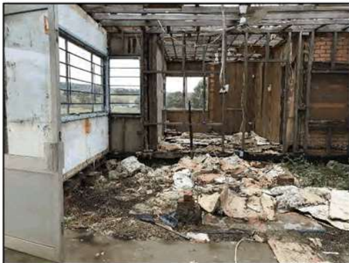
Figure 28. View to the interior of the former hardware store as viewed from within the building, facing north. Note the caved in roof and extensive damage within the building.
