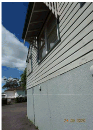
Figure 4.15 Detail view of northern elevation showing the contemporary awning on the rear windows and cracks in the foundations.
