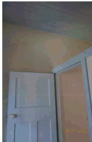
Figure 4.58 Detail of the partition wall and door leading to rear study showing beam and high ceiling.
