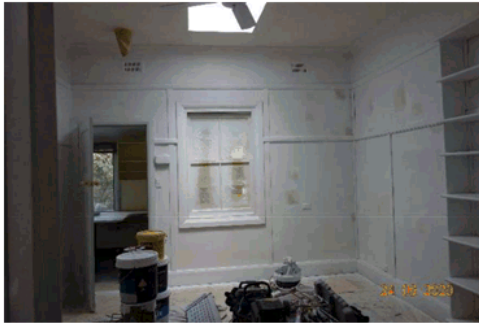
Figure 4.35 Typical view of a modified interior room with original timber details, and contemporary ceilings, fixtures and joinery.
