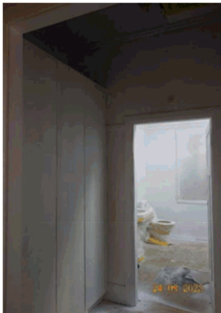
Figure 4.37 View towards the bathroom from the corridor showing later joinery, facing south.
