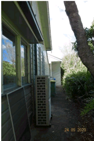
Figure 4.13 View of the southern elevation showing the contemporary louvered windows and guttering, and the concrete access path.
