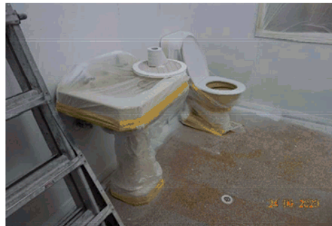
Figure 4.38 Detail of mid-century bathroom fittings and contemporary flooring and skirting.
