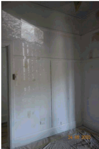
Figure 4.25 Detail of timber finish on the southern wall and skirting boards in entrance foyer.
