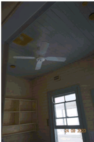
Figure 4.57 Detail of the painted timber ceiling and rear wall between enclosed rear verandah.
