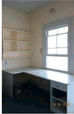
Figure 4.56 Inset desk facing northeast and window to enclosed rear verandah. Detail of the partitioned area of the rear weatherboard extension with fixed furniture and joinery.
