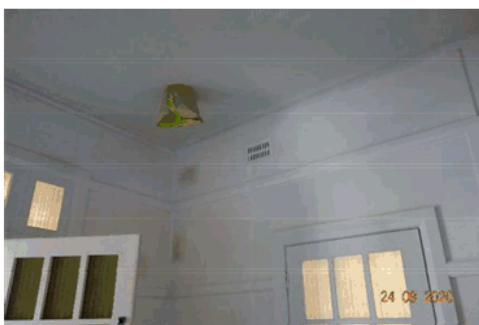
Figure 4.23 Entrance foyer (looking northwest) showing ceiling with a contemporary light fixture covered by plastic.
