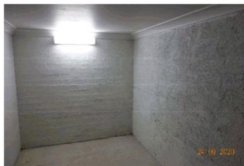
Figure 4.54 Detail of the southwestern corner of the basement showing the rendered interior of the external walls
