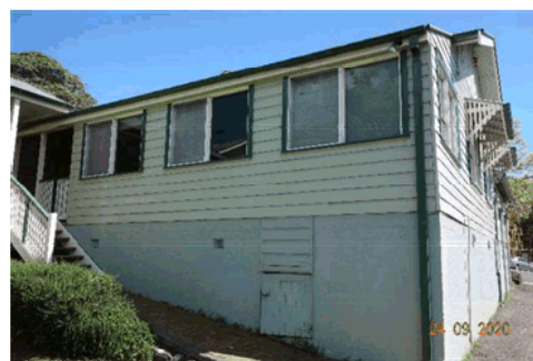
Figure 4.18 View of the rear (eastern) elevation with enclosed verandah and aluminium-framed windows.
