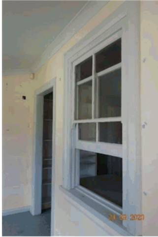
Figure 4.55 Detail of the window and door leading to enclosed rear verandah. The window appears to be original.
