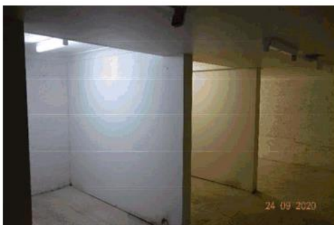
Figure 4.53 View of the partition walls in the rear area of the basement. The rising damp on the partition walls can be seen.
