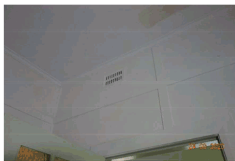
Figure 4.30 Ceiling and joinery in the front room showing wall detail and original vent.
