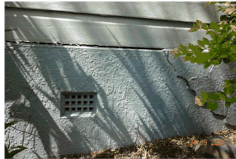
Figure 4.20 Detail of the foundations on the western elevation, showing cracking and areas where the weatherboard is lifting
