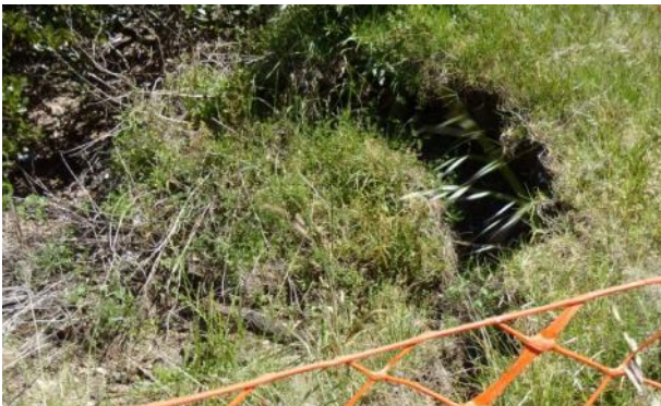
Site 9 – Riverside Drive stormwater scour
