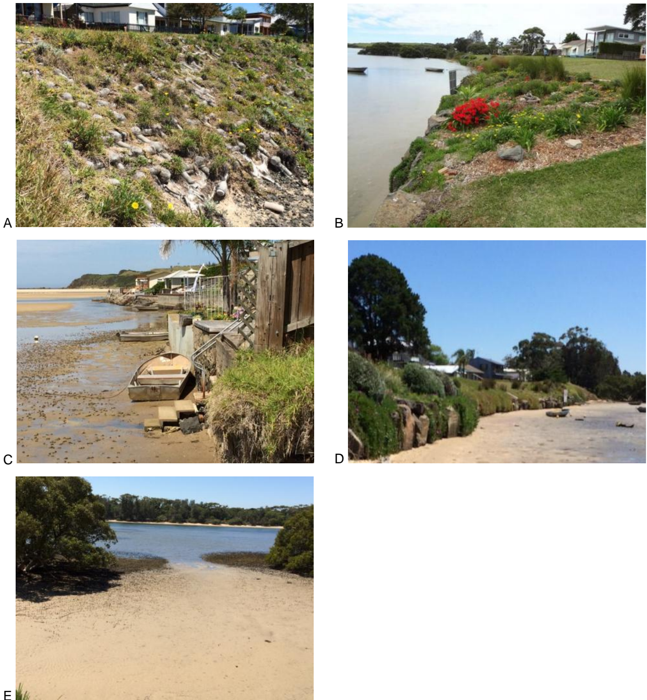
Figure 30: Charles Avenue erosion and existing controls
