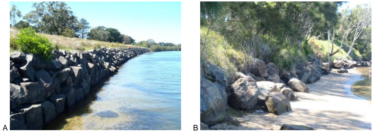
Figure 31: Riverside Drive erosion controls
