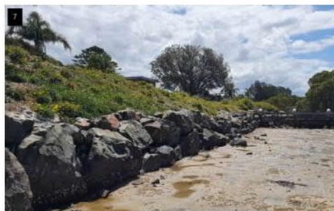
7. Rock wall with mix of large (~600mm diameter) and smaller rock. Scour along crest of wall. Areas of exposed concrete matting and geotextile. Slumping in some sections. Grout has been applied along the crest in some areas. Increase height of wall or add additional scour protection along crest. Rebuild/recycle existing rock. Install rock scour protection along toe to prevent future slumping/overturning
