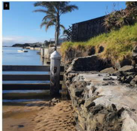
3. Grouted rock wall approximately 1m high. Necking of timber groyne piles - repair with a concrete filler collar (FRP collar that wraps around the pile and filled with appropriate mortar mix) or similar.
