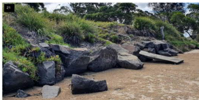
21. Concrete ramp with lower portion made from FRP. In good condition. Displacement of rocks either side of ramp and minor slumping - increase height of wall crest.
