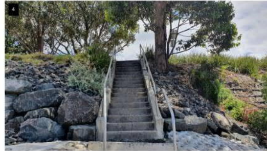
4. Mixture of small rubble and larger rock. Staircase experiencing settlement and cracking. Large gum and light pole at top of stairs. Crest level approximately 3m AHD. Rebuild staircase on stable foundation or on piles. Rebuild revetment (retaining tree as bank stabilisation) with rock rip rap to an adequate scour depth. Vegetate with sprawling pigs face, alternatively a salt marsh berm can be incorporated. Retain light pole and shower if possible, alternatively replace with solar light and move landward.
