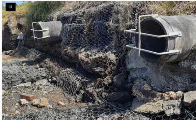
13. Two reinforced concrete storm water pipes. Gabion scour protection. Gabion baskets have been repaired and some are in need of repair. Consider replacing gabions with stone blocks in the future.
