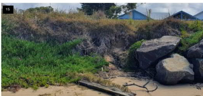
15. Slumping of bank adjacent to rock protection. Continue rock protection all the way along bank to ramp.
