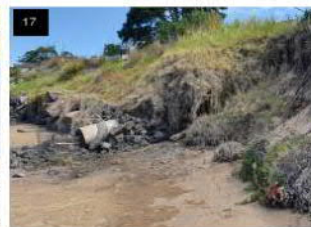
17. Two reinforced concrete storm water pipes with gabion scour protection. Slumping occurring next to the pipe at approximate CH 510, continue rock wall in this area. Repair displacement and cracking of storm water pipes. Add rock scour protection.
