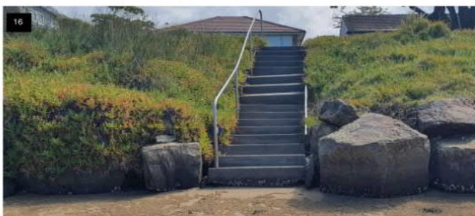
16. Rock wall approximately two stones high, well vegetated and in good condition from CH 400 to CH 500. Concrete stairs showing signs of displacement. Consider toe scour protection along extent of rock wall.
