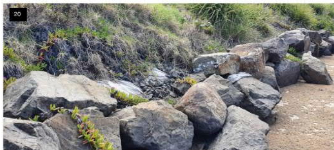
20. Erosion occurring along crest of wall. Wall height needs to be increased. Displaced rocks along extent of wall - better placement required. Rebuild wall (approx two stones high) and rock scour protection along toe.
