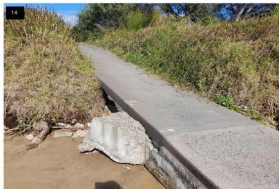
14. Concrete ramp exposed at toe and experiencing washout underneath. Erosion occurring along the downstream bank. Cutoff ramp above HWM and replace with FRP mesh on piles at end.
