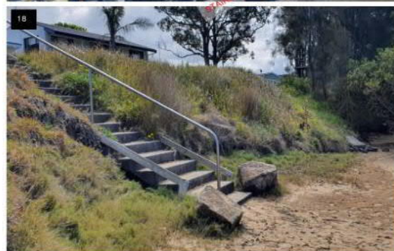
18. Concrete stairs currently in good condition. Displacement may start to occur in sections where material is being washed out from underneath. Fill under concrete stairs with concrete. Add rock scour protection at toe or alternatively place on piles.
