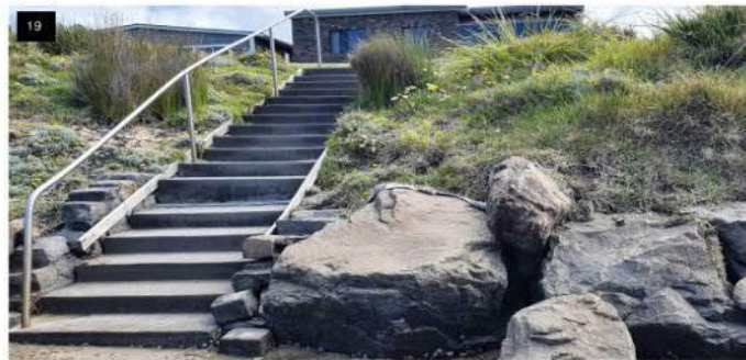
19. Minor settlement of stairs occurring. Grout has been used on the stair landing aimed at minimising further settlement. Rocks placed either side of stairs as scour protection. Material appears to be being washed out from under stairs. Replace lower portion of stairs and place on piles.
