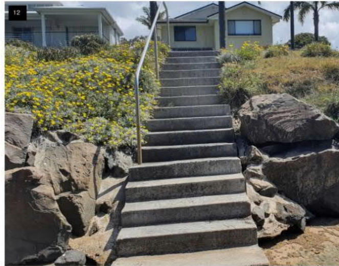
12. Concrete stairs experiencing minor settlement. Rebuild lower section of stairs on piles.
