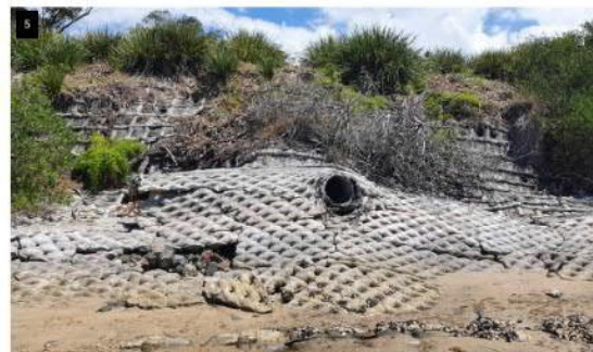
5. Deteriorated concrete storm water pipe with exposed reinforcement. Displaced and cracking concrete mattress. Washout of bank behind mattress. Remove concrete scour matting and construct revetment as in point 4.
