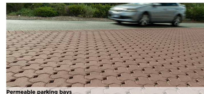
Permeable parking bays
