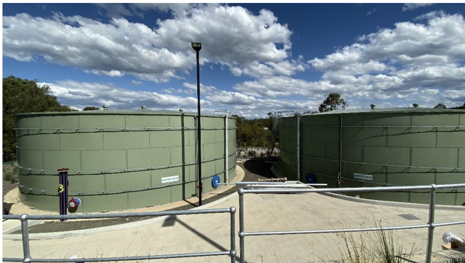
Figure 5 Example of Drinking Water upgrades required for growth in Springside Hill (refer to Appendix A for proposed location)
